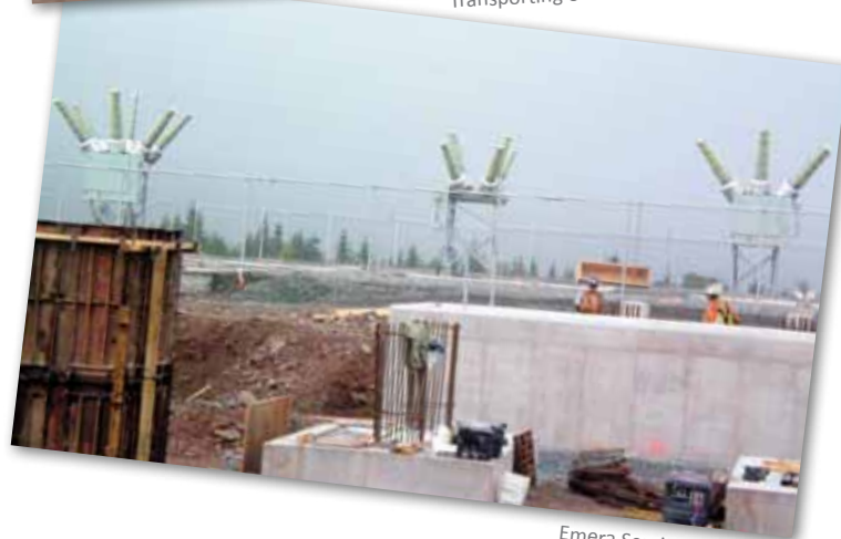
Emera Service Substation
